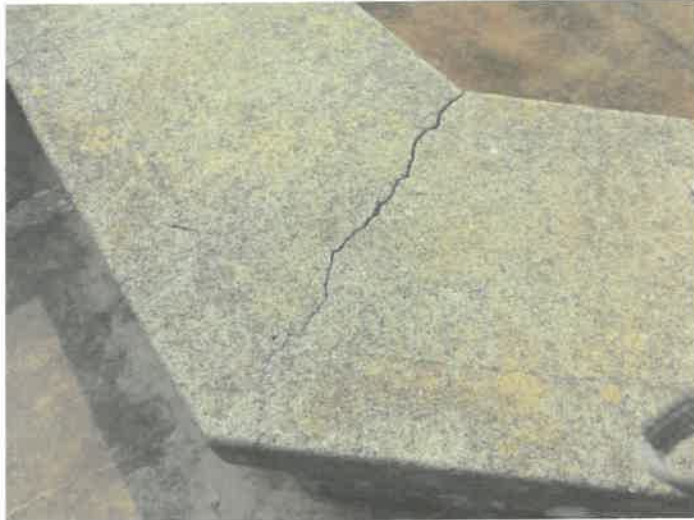
Figure 48 – Corner crack in Terrace railing
