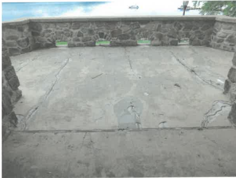
Figure 29 - Floor cracks in Park level slab, looking south at the Terrace
