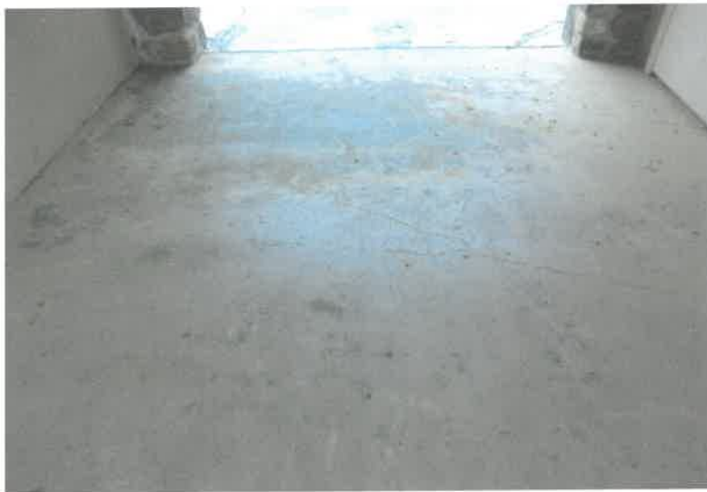
Figure 33- Floor cracks in Park level slab (tunnel) looking south
