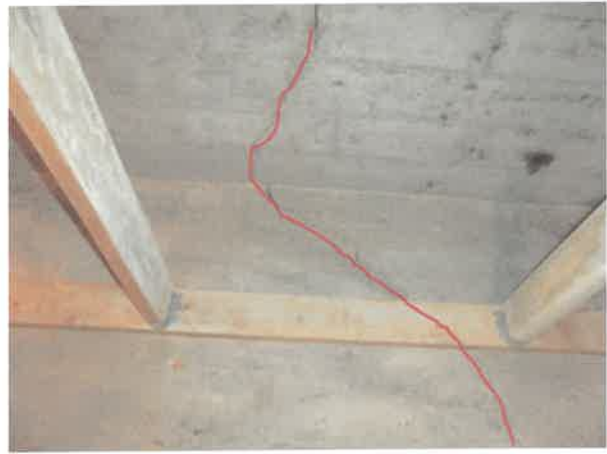
Figure 21 – Wall crack in Figure 20 continues into the slab above
