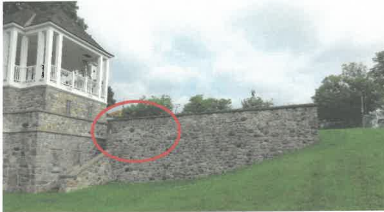
Figure 72 – East retaining wall showing efflorescence.
