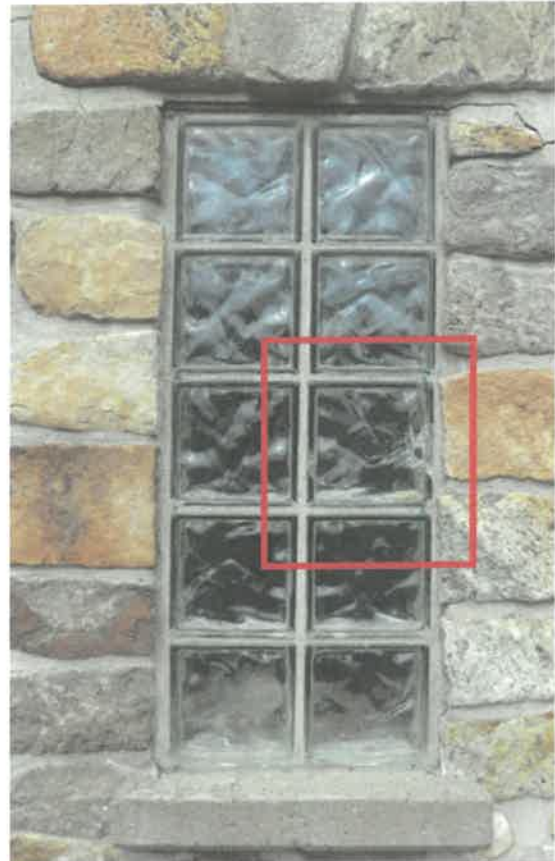
Figure 37 – East wall, broken glass block
