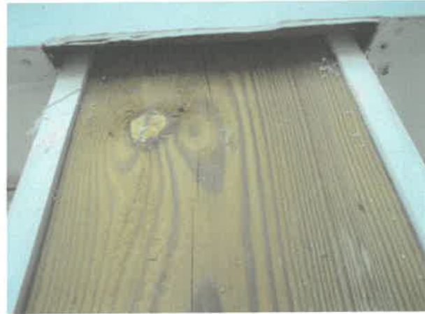
Figure 57 – Removal showing no strap at top
