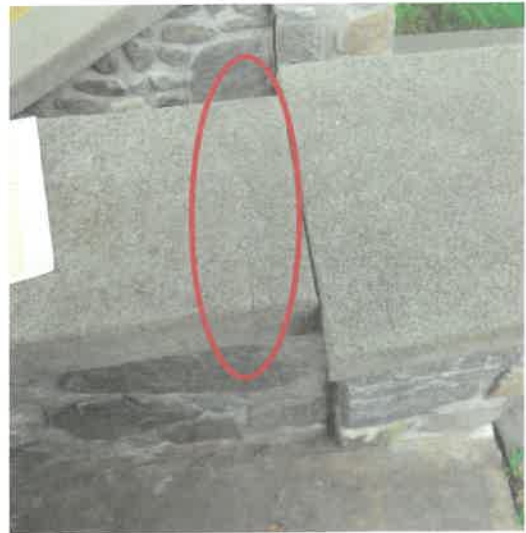
Figure 49- Crack in railing cap near the west stairs
