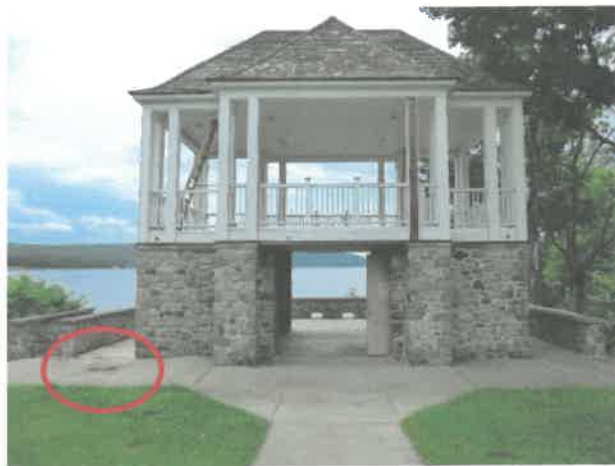
Figure 73 – Shows the catch basin
