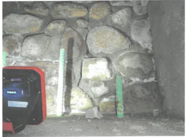
Figure 11 – North Wall crack
