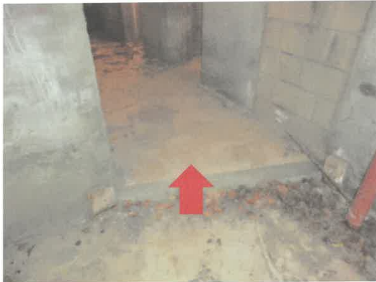
Figure 24 – Overpoured concrete floor
