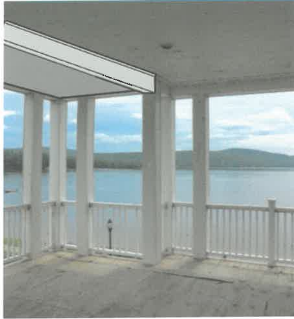
Figure 78 – Possible dropped beam in the ceiling
