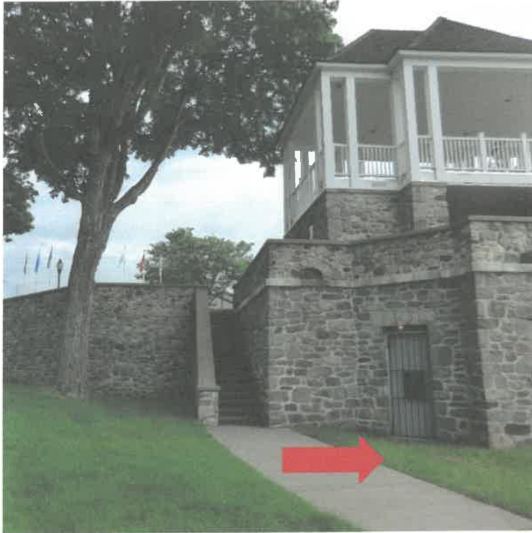
Figure 77 – Tree roots adjacent to building
