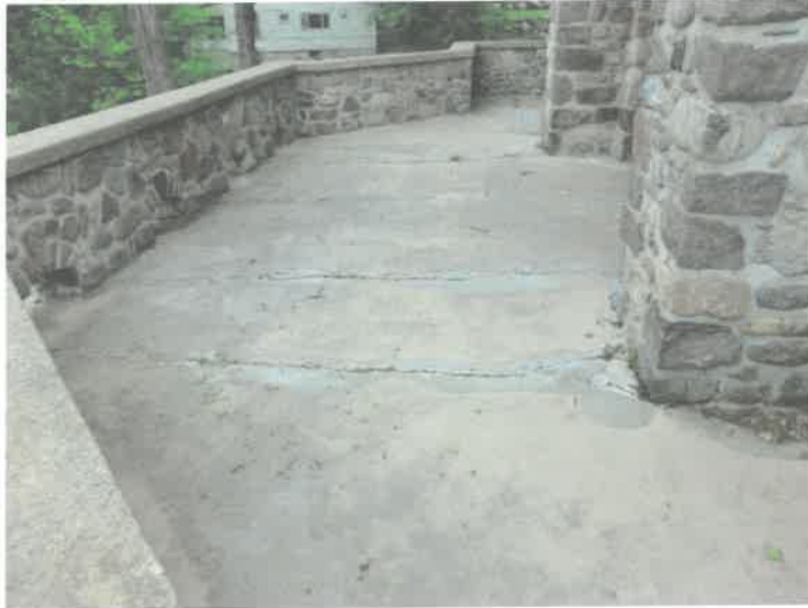
Figure 32 – Terrace cracks looking west
