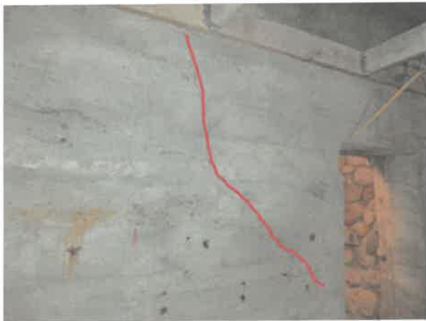
Figure 20 – Interior wall crack
