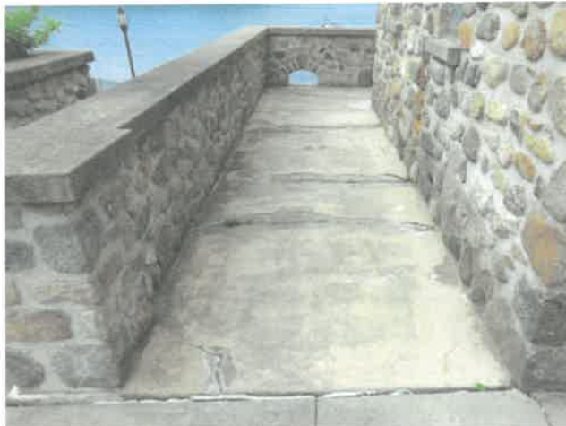
Figure 30 – East walkway cracks
