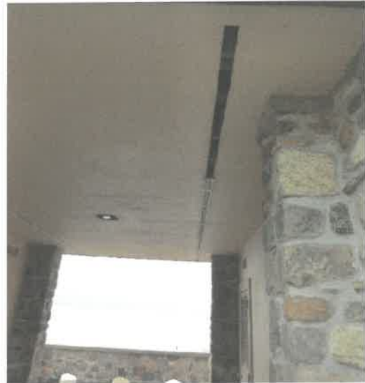
Figure 40 – Missing and damaged vent
