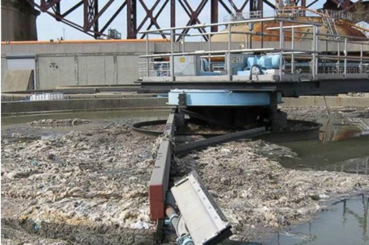
Wipes clogging a wastewater treatment clarifier. These clarifiers are for sedimentation of particulates to separate the sludge from the water – there should be no visible debris on the surface. Photo courtesy of City of Vancouver, WA.
